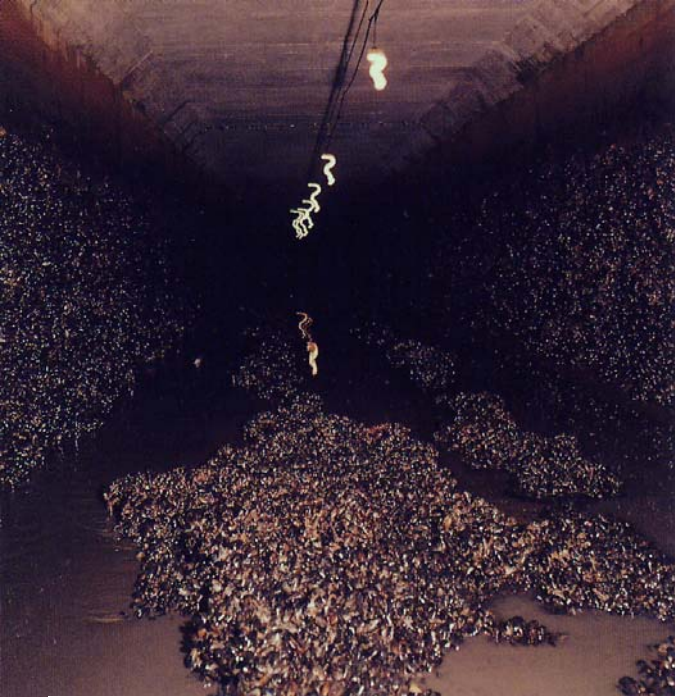
Mussel fouled power station culvert
